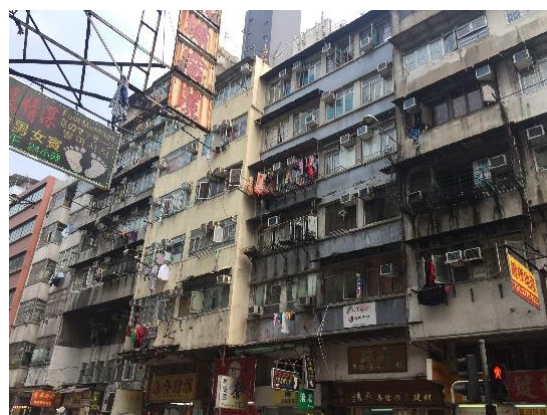
Poor Building Conditions 不良的樓宇狀況
